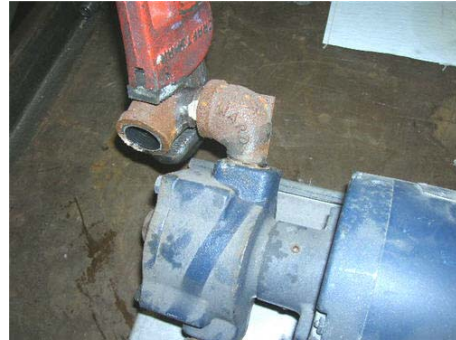
Step 16 Remove one of the two 90 degree 3/4" npt street elbows from pump head outlet piping by using an adjustable pipe wrench.
