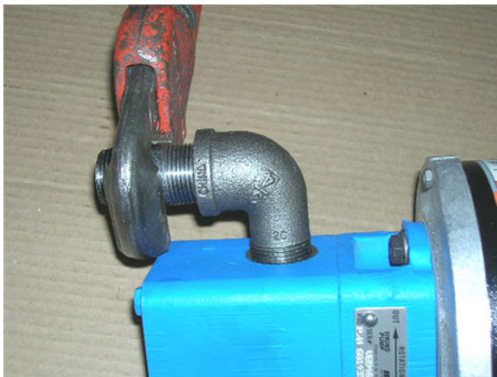
Step 16A. (Viking Pump Replacement Only) Remove 3/4" npt space nipple using a large adjustable pipe wrench.
